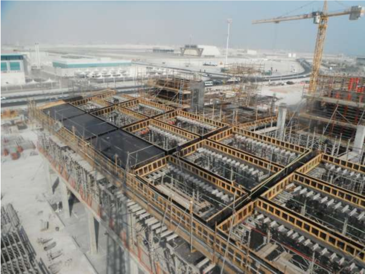
View of the Backup Approach & Training Center Building during installation of roof formwork
