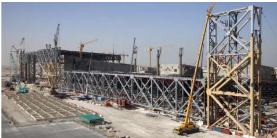
Aircraft Hangar -The roof of the smaller hangar has already been lifted to its final position. The roof of the larger hangar is still being assembled.
