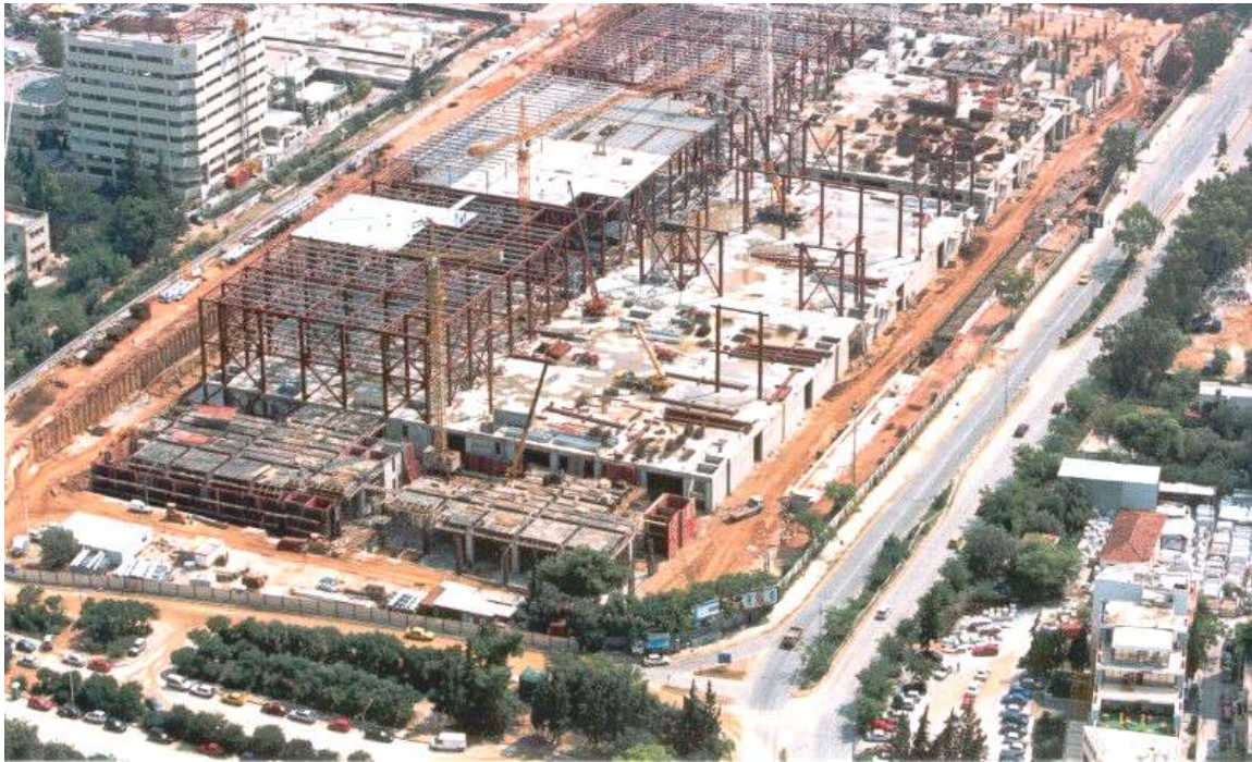
International Broadcasting Center: Completion phase of the concrete structures and initial assembly stage of the steel structure
