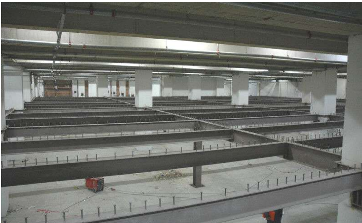
Post-Olympic addition of a middle floor in the lower part of the IBC building, for the provision of additional car parking
