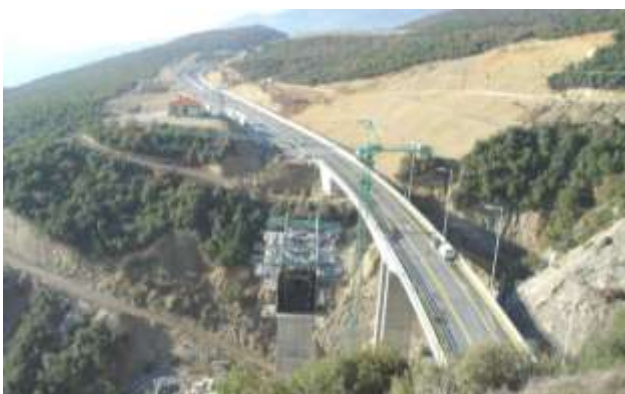
Bridge Γ2: The construction of the right branch has been completed - The left branch is under construction
