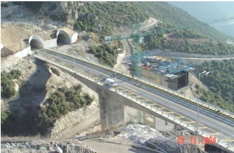
Bridge Γ1: The construction of the right branch has been completed - The left branch is under construction
