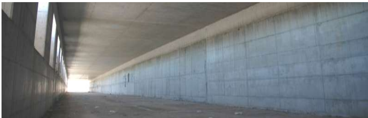
Completion of concrete works of the single cell Cut & Cover tunnel, 450.0m length between km 14+540 and 14+950
