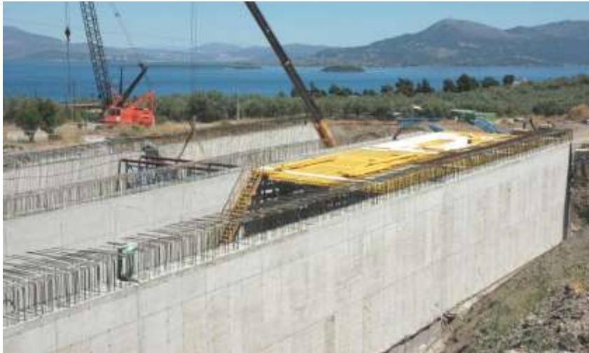
Part of the Cut & Cover tunnel at chainage 11+824.0 during the roof construction phase
